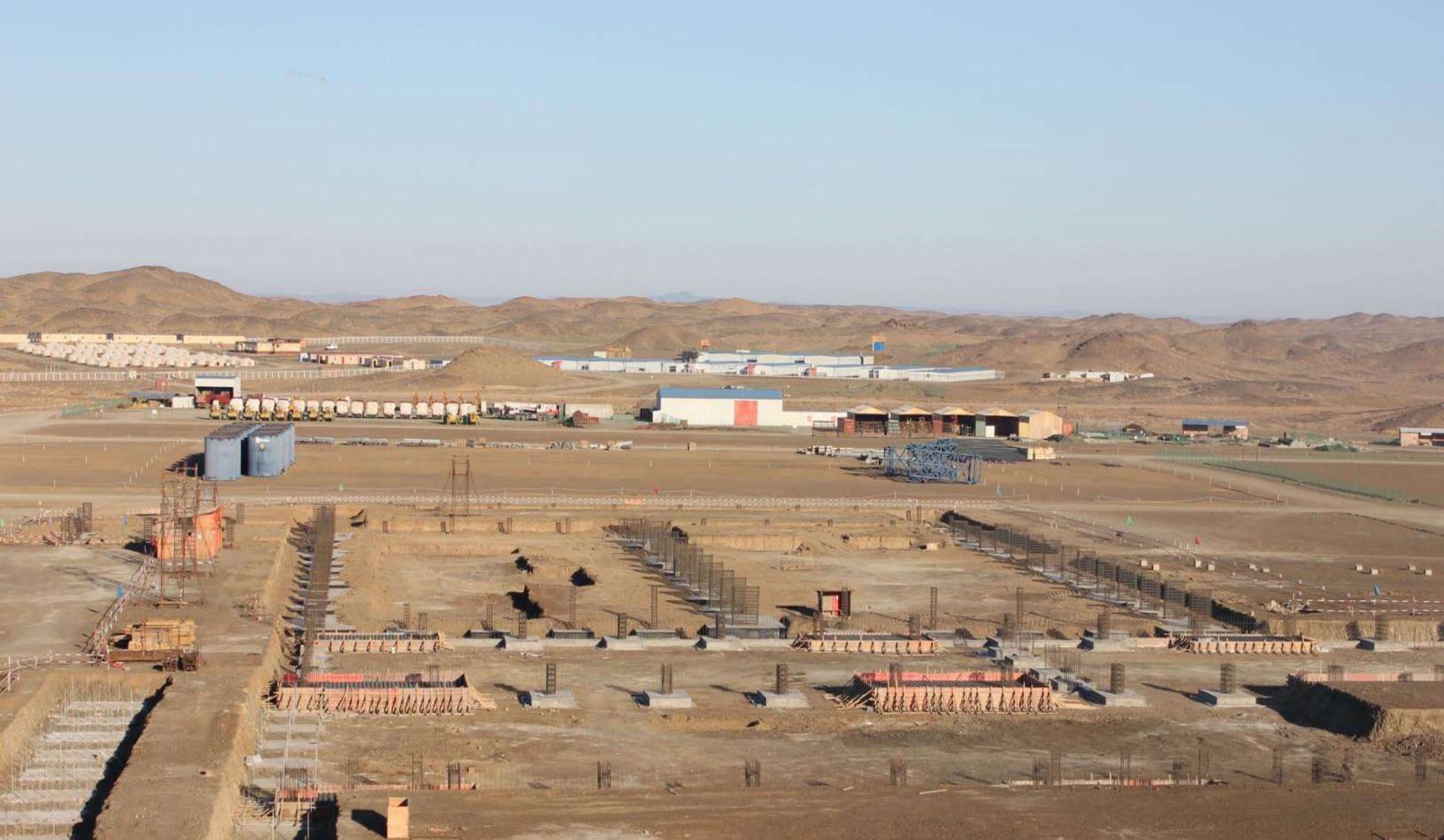
Flotation and filtration building
